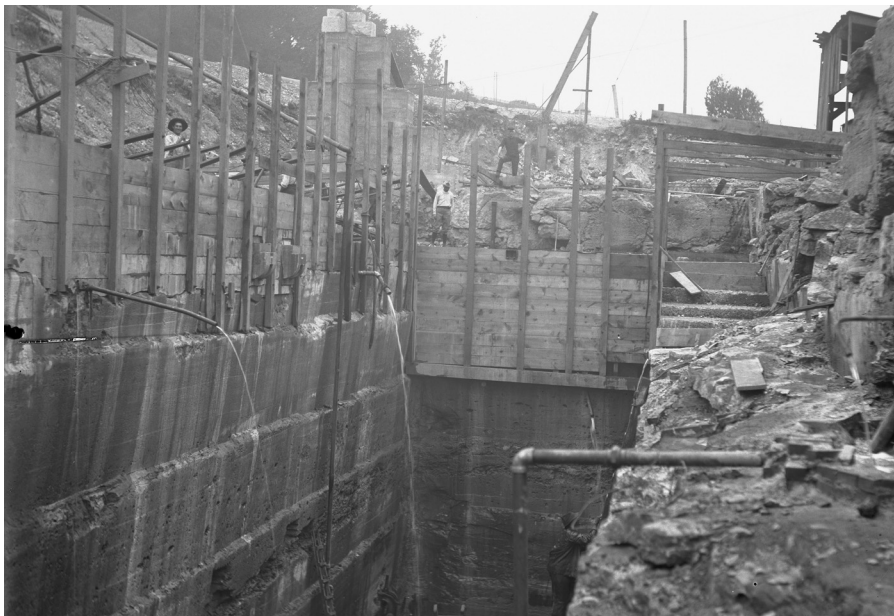
The wheelpit for Rankine had to be excavated to a depth of 171 feet below the generating station floor, with an opening almost 567 feet long. Unlike conventional open-pit or quarrying operations, the sides had to be close to vertical. Compressed air from a steam-powered compressor plant at the surface powered the drilling and cutting equipment.
