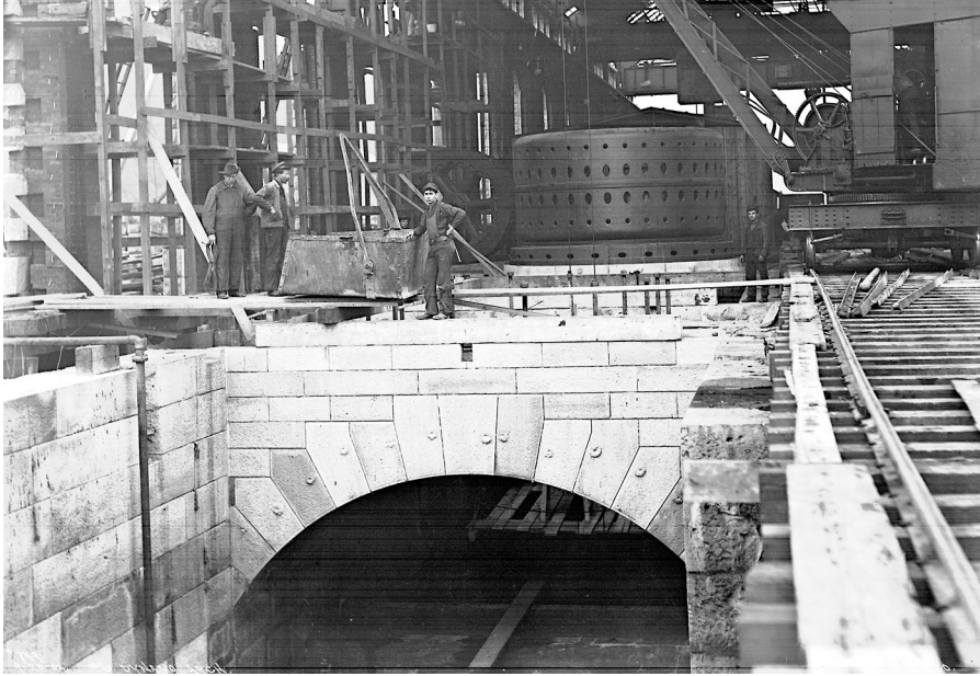
The Rankine generating station features 11 generator arches made of stone and heavy cast-iron structural elements that span the wheelpit. The generator in the background of the photo is resting on a completed arch. Floor plates between the arches are removable to allow turbines and other equipment to be raised up from the wheelpit to floor level for maintenance and repairs.
