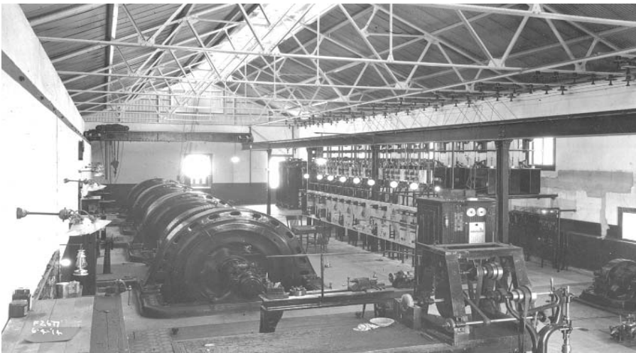
The Santa Ana River No. 1 powerhouse was rewired and a marble switchboard was installed in 1914. The powerhouse was designed to hold six turbine-generator units, yet only four units were installed. The additional units would have occupied space at the west end of the building, shown in the foreground of this photo.
