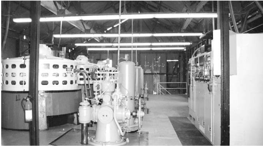
The plant sat idle for 30 years after it was nearly destroyed by flooding. In 1990, Jimmy Parker and his wife Linda rebuilt the facility. Modern switchgear was added. The generators, governors, and turbines were completely refurbished, upgrading the plant to 1.4 MW. In the winter of 1993, the Cuero hydro plant was back in operation.
