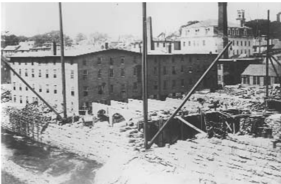
This photograph, taken in 1894, shows construction of the Bridge Mill Power Station on the Blackstone River. When it was developed, engineering publications called the project the “finest water-power electric station in New England.”
