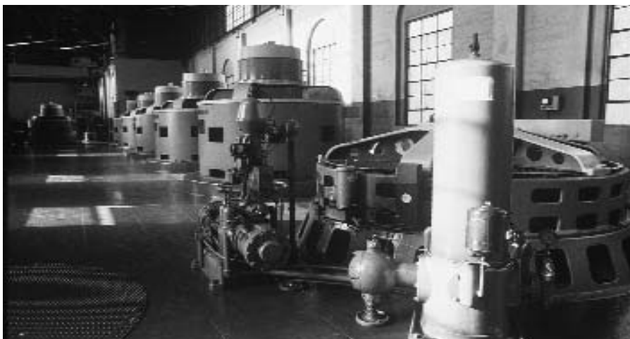
The turbine deck at Portland General Electric's 16-MW T.W. Sullivan hydroelectric plant, as it looks today. In addition to producing power, the plant's innovative fish screen and a new fish evaluator system are providing useful data for fisheries research and management.
