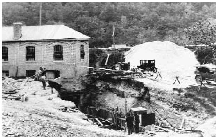
This photograph (circa 1920) shows construction under way on the outlet flume at the Lanesboro, Minnesota, hydro plant. A second turbine-generator added at this time doubled capacity to 480 kW to meet rapidly increasing electrical demand.
